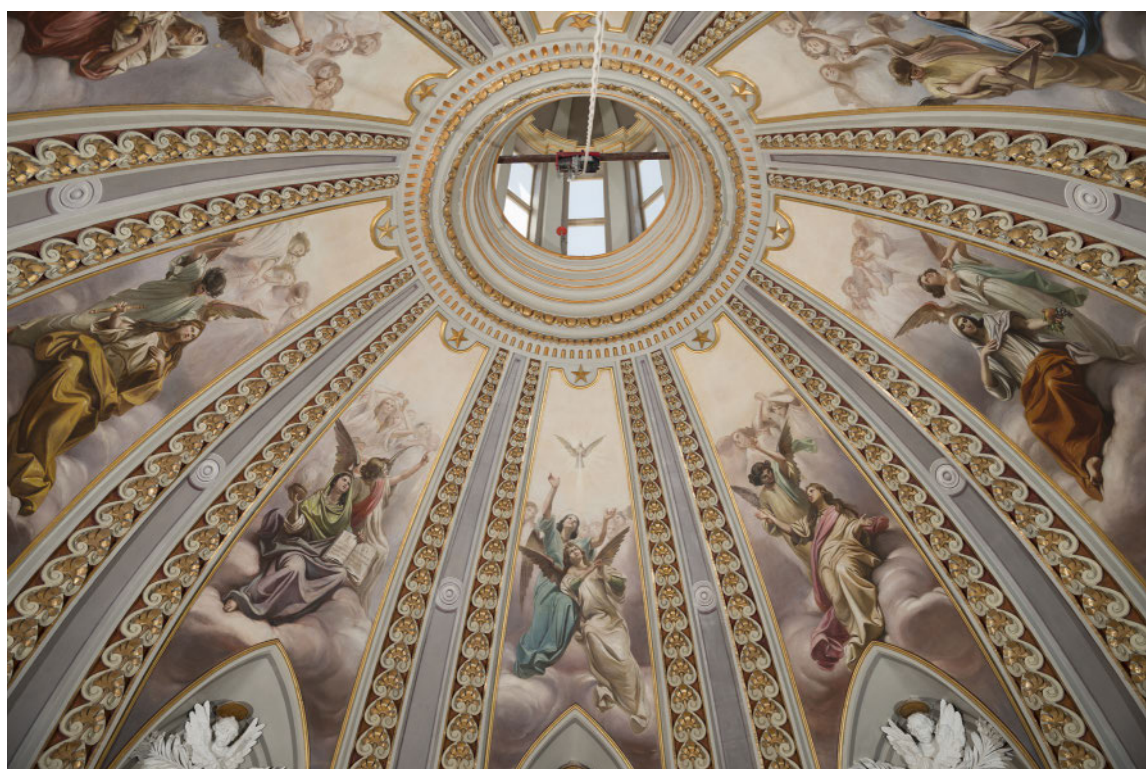
Half dome of the Basilica of Our Lady of Porto Salvo and St. Dominic, Valletta, Malta. After conservation by Agatha Grima Conservators. Image courtesy of Agatha Grima.
