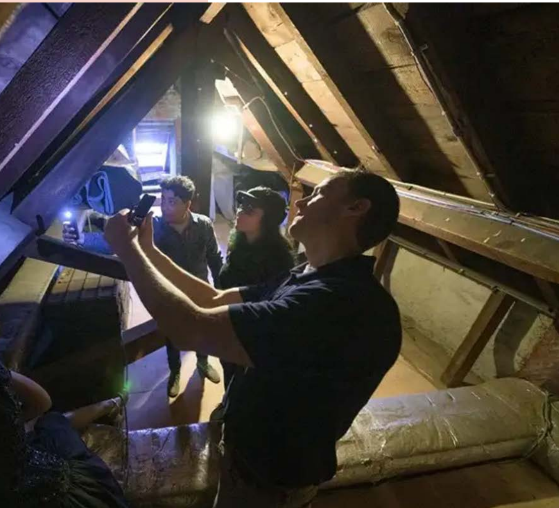
Above: In the museum's attic, team members (from left) Margalit Schindler, Morigan Kelley and Tim Leefeldt check out the condition of some wooden beams. Image by Evan Krape / University of Delaware
